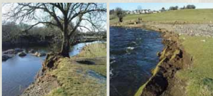
Examples of bank destabilisation on Paplava Farm at Cockermouth following flooding in 2009
