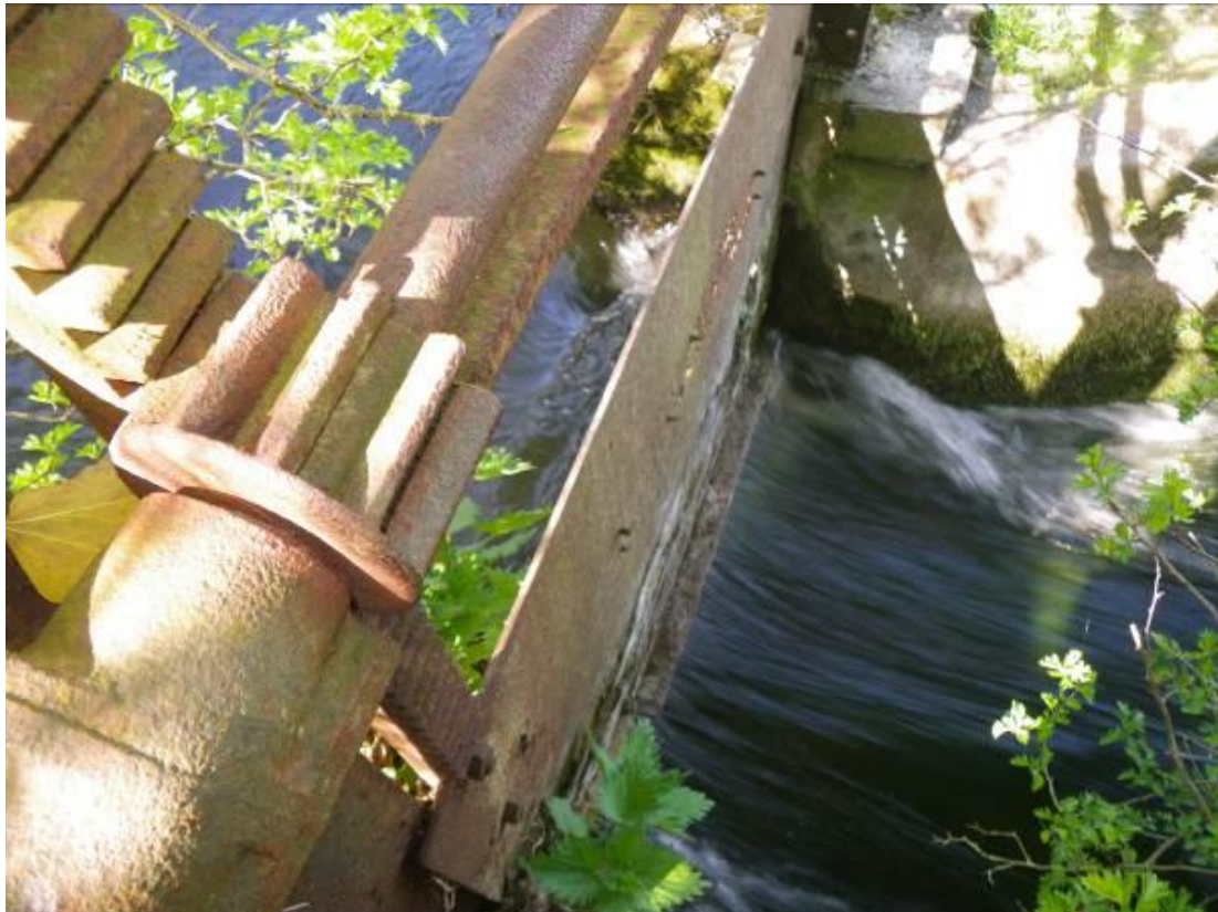
Photo 1. Single undershot hatch at the head of the Elm Stream. A barrier to fish migration.
