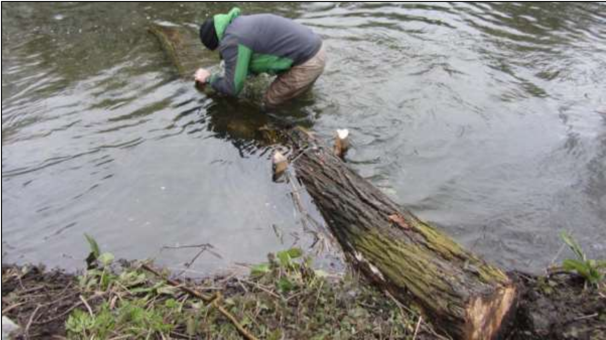
Figure 6: A simple log deflector installed pointing upstream and keyed into the bank will deflect flow out into the centre of the channel.
