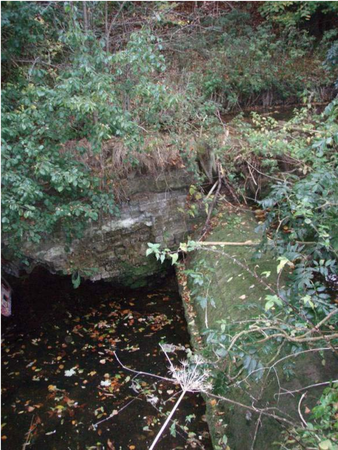
Photo 11 Brick weir / sluice structure – a significant barrier to fish movement and an obstacle to re-colonisation of the river following the 2008 pollution.
