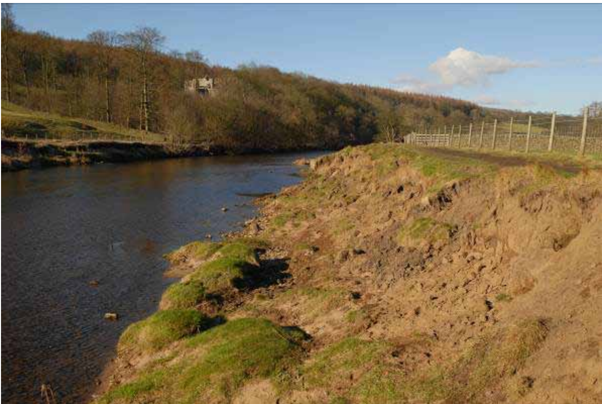
Erosion on River Wharfe looking u/s to Barden Bridge
