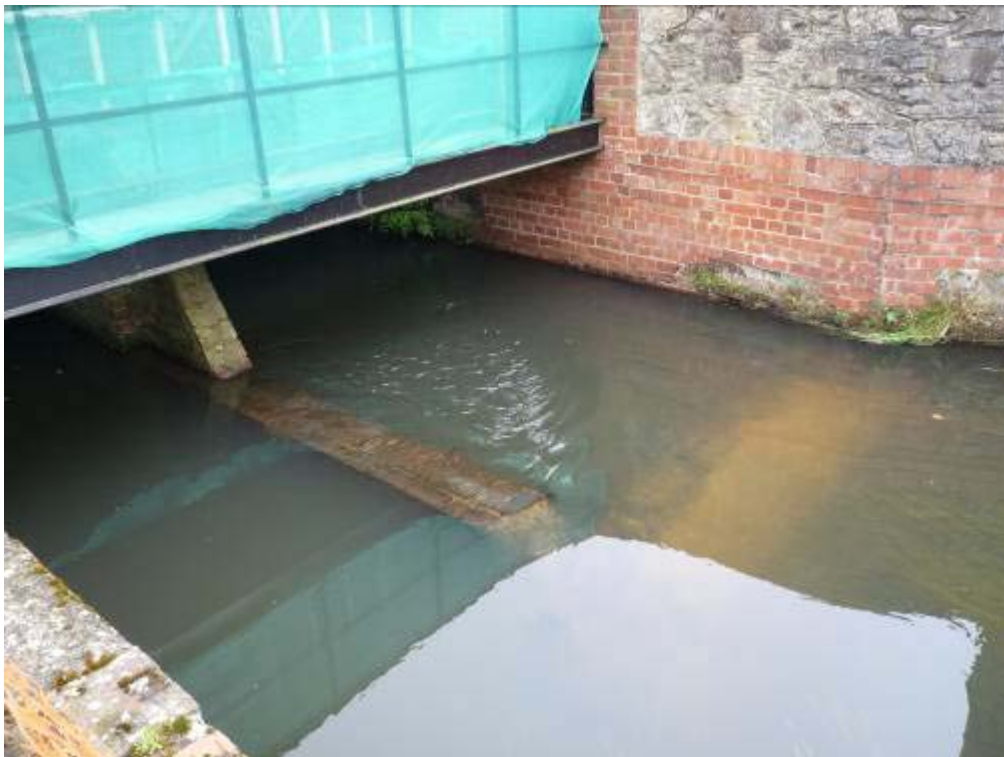
Entrance to the hatches. Note the presence of ribbon weed in mid channel.
