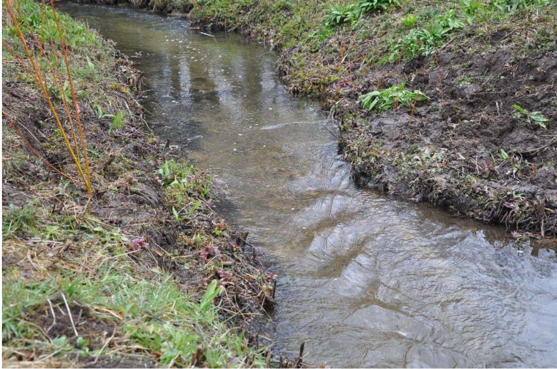
Photo 13 Simple bank re-profiling to pinch the channel. The front edge of the new bank could be defined with brushwood bundles before re-profiling.
