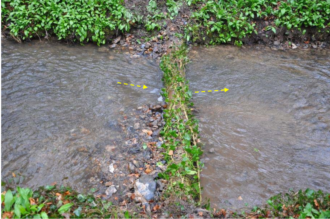
Photo 9 A cross-channel log, keyed into the bank and set at or just above bed level, with a narrow channel excavated (yellow arrow) beneath to promote bed scour. Excavated material is placed at the sides against the bank.
