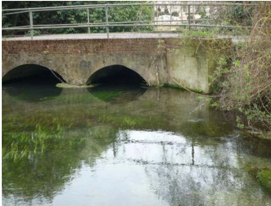
Road bridge at the bottom boundary. Lowering the bed level beneath the right hand arch should promote increased velocities in the bottom of the carrier
