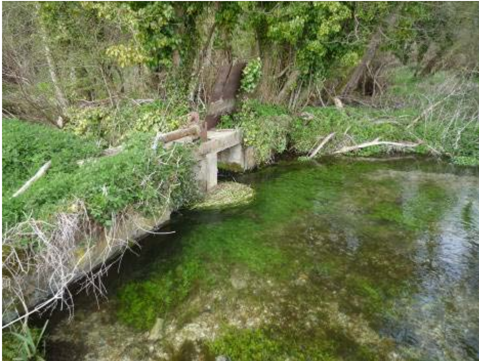
Old water level control hatch – Is it really needed?
