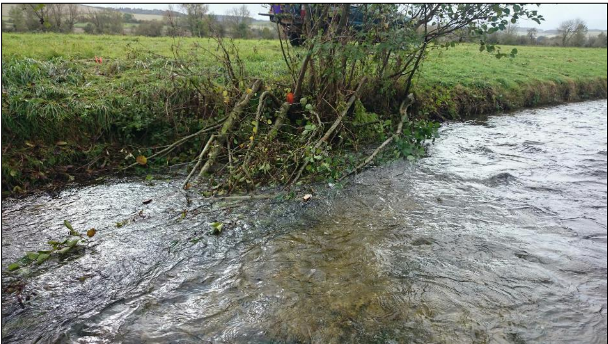
Figure 21: Small limbs 'hedge-laid' into the river and secured with stakes (cut off below water level)
