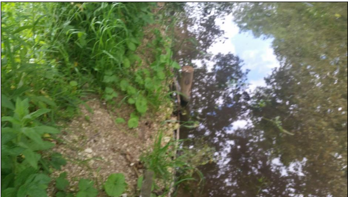
Figure 10: Gravel on top of the brushwood provides good long-term transitional habitat and bank protection
