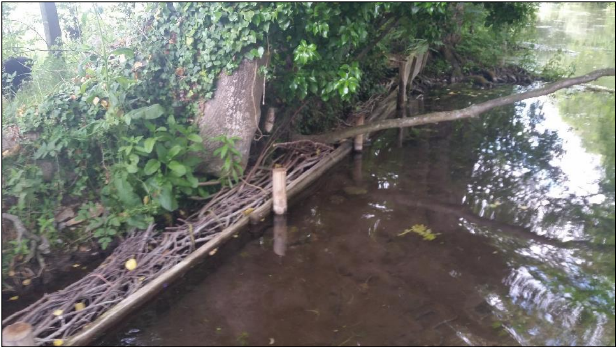
Figure 9: The wooden shuttering is in the process of being replace with brushwood faggots
