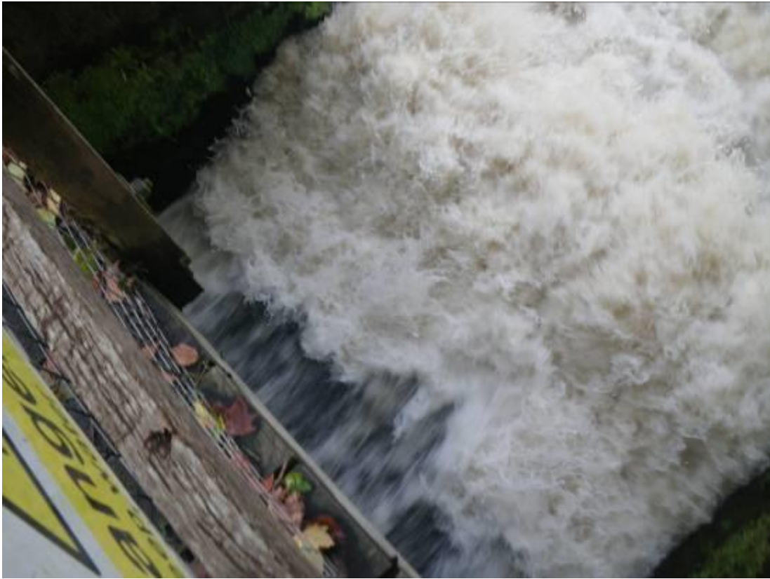
Photo 3. Under shot weir gate at Stedham. A sea trout was observed jumping at this structure on the day of the visit and failing hopelessly to make any upstream progress.
