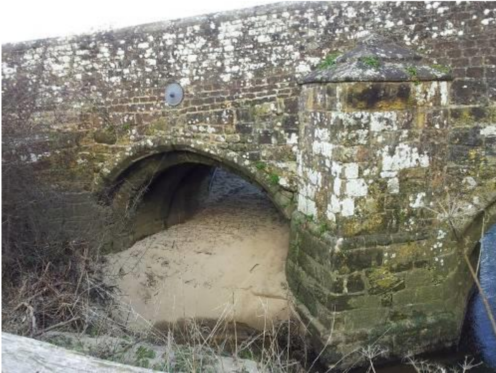
Photo 1. Sand deposited under Woolbeding Bridge. A Rother speciality!
