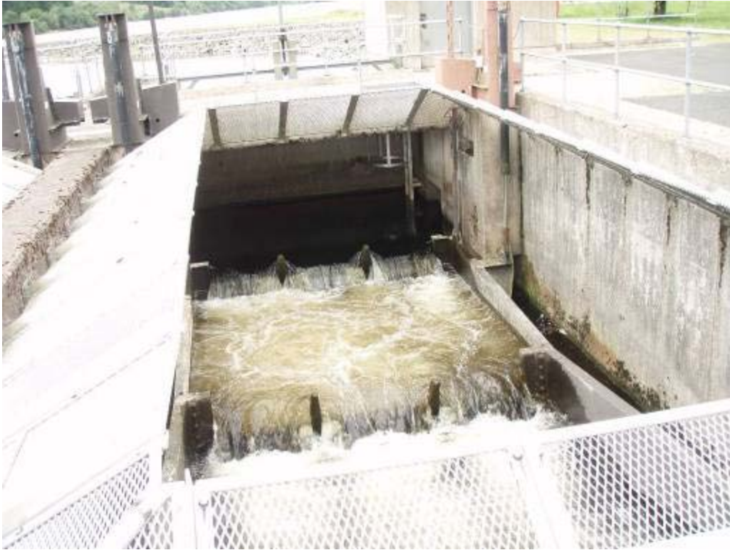
Photo 3 Outfall arrangement at head of one of two concrete culverts (loch in background)
