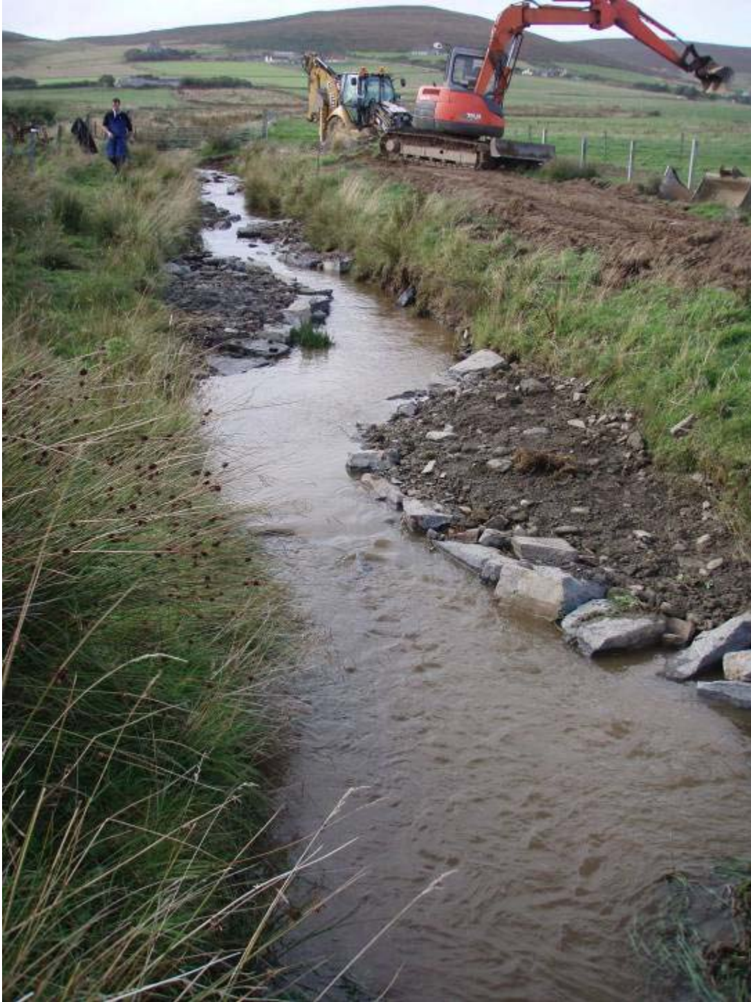
Photo 16 D-groynes installed on an burn on Orkney. In the absence of grazing, these vegetate quickly. Their low profile allows flood flows to overtop the structures.
