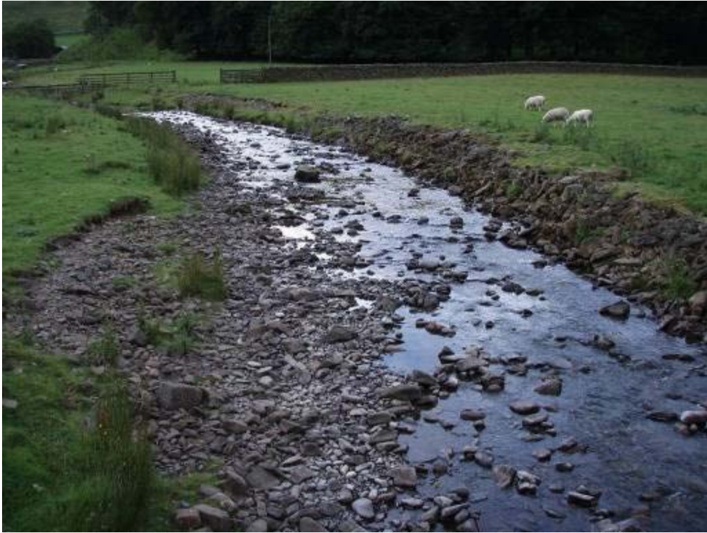
Photo 10 Crosscleuch Burn. Overwide channel, modified to provide bank re-inforcement. Lack of depth variation and no pool structure.
