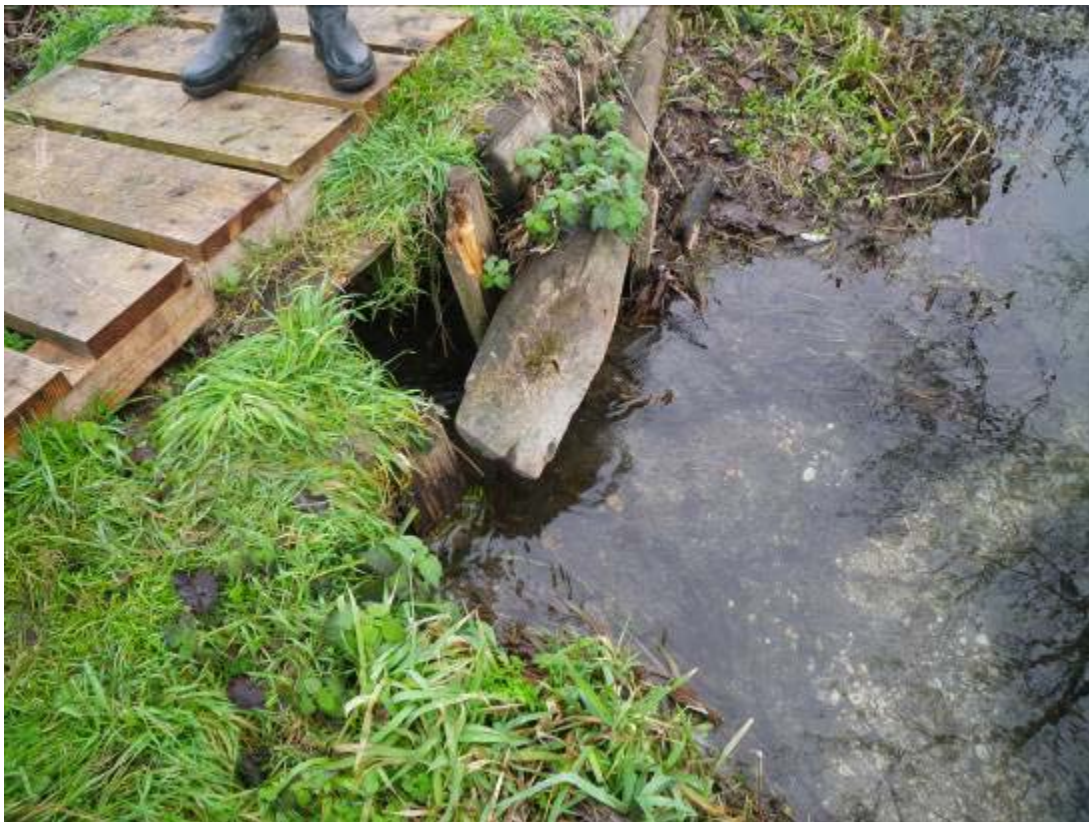
Water being lost to the meadow via a bank breach which was possibly the site of an old structure
