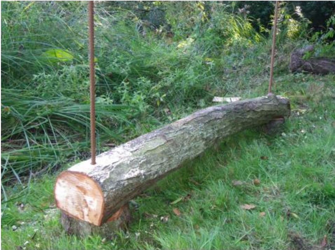
Photo 10. Cover log sat up on two woody rings cut from the end of the log, drilled and ready to be pinned to the bed with steel re-bar.
