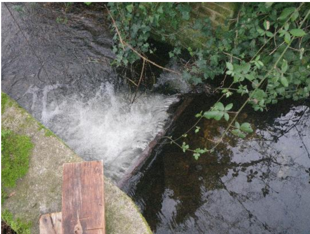
Photo 7. Water level control boards at the head of the by-wash channel.
