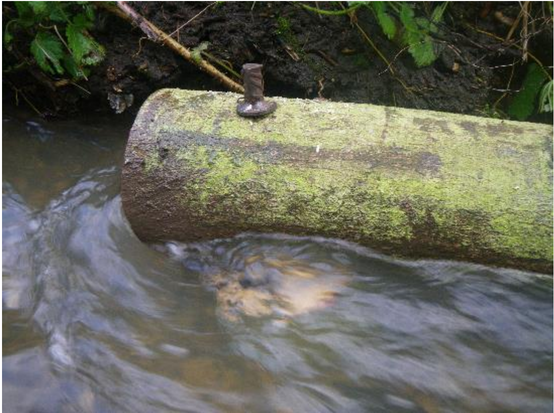
Photo 11. Correctly installed parallel to the flow and tight against the river bank.
