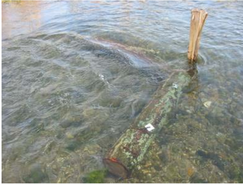
Paired LWD limbs used to create a 'v' shaped deflector. Note rebar and steel washer fixing
