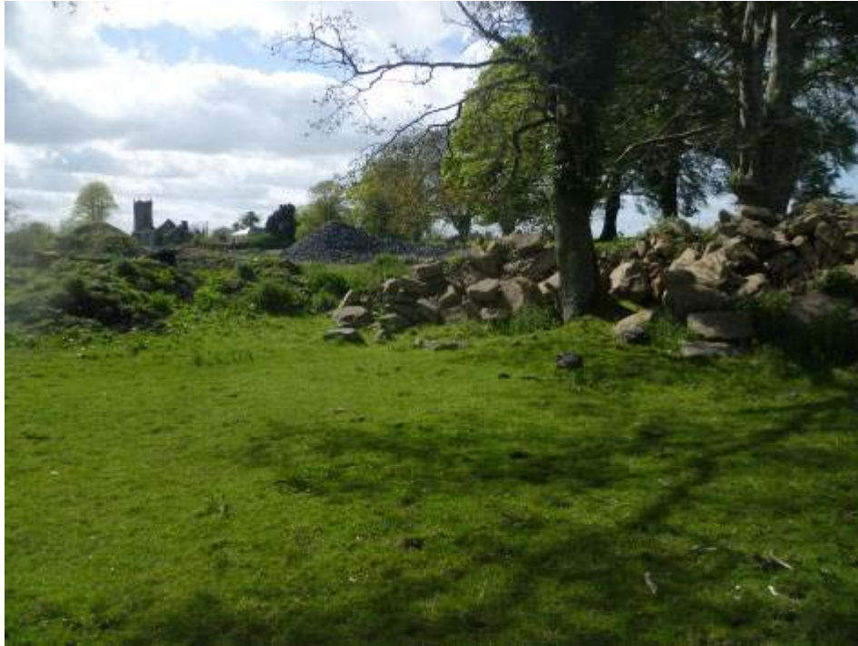
Stone/gravel piles on RB upstream of Crossboyne Bridge
