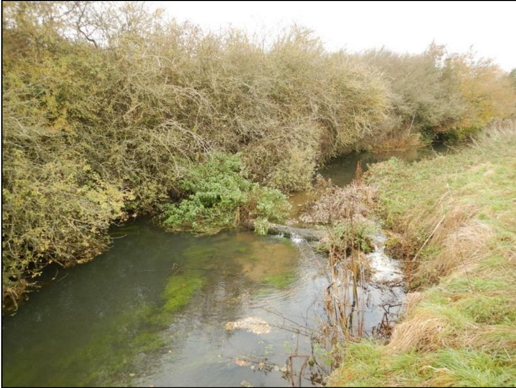
Pic 21 (TL 39254 23656) – The weir, which instead of focussing flow in the centre of the channel, is now causing bank erosion and impounds the reach above it.
