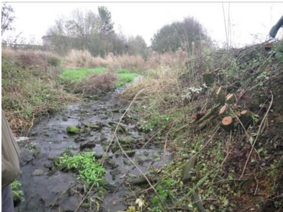
Photo 2. The downstream face of the ford structure looking up towards the top of the structure.
