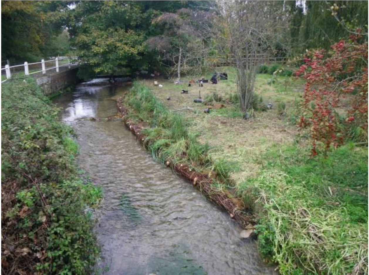
Photo 5. A new bank toe created using faggot bundles plus a gravel in-fill and planted with aquatic emergent plants. If properly constructed, a bank like this is hugely resilient and will protect the foundations of the existing hard wall (now obscured from view). The new toe also creates a valuable new habitat.
