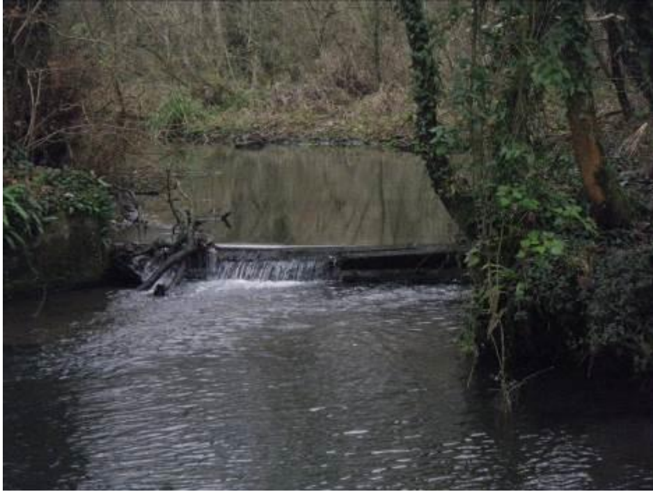
Photo 1. Small weir at the top of the reach could delay fish migration in a dry autumn and will be adversely impacting on upstream habitat quality.
