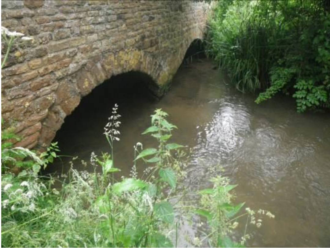
Photo 1. The downstream side of Woodford Bridge. The limited capacity of the bridge and potentially bed armouring underneath may be responsible for sedimentation issues on the reach above.
