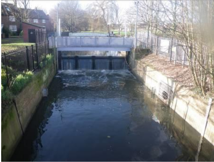
Photo1. The weir located on the Crane at the bottom of Knellor Gardens. The structure appears to block upstream fish migration via this route and is a serious impediment to habitat restoration in the reach immediately upstream. The headloss may be reduced when high spring tides coincide with strong fluvial flow.
