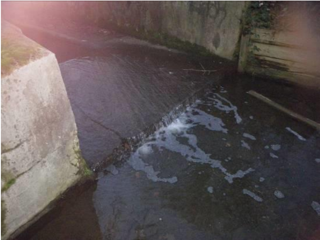
Photo 6. Another box section on the tail of this structure is required to enable fish to swim up to the next step.
