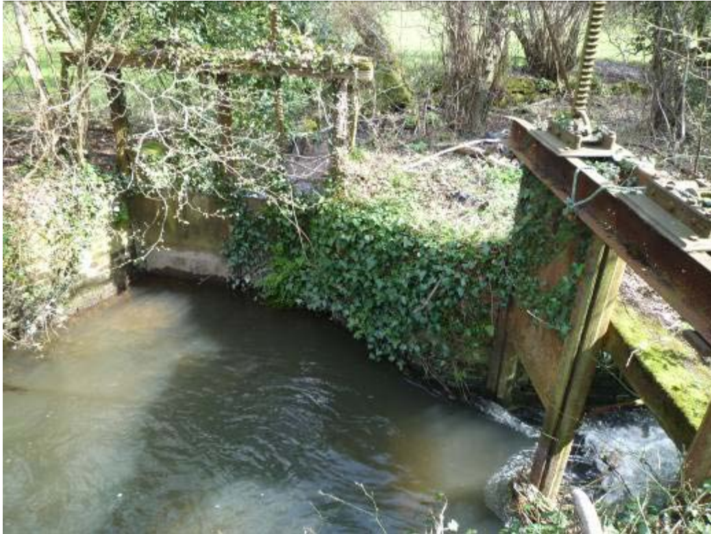
Old water meadow hatches with the main structure fully drawn and the drowning gate fully closed
