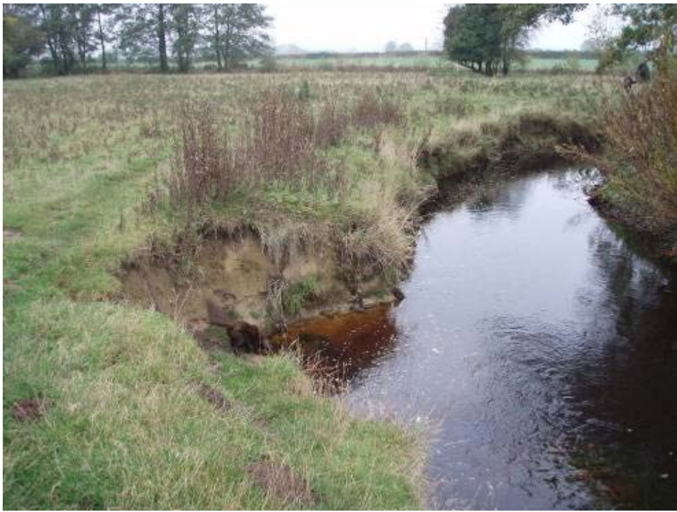
Photo 5 Limited areas of bank erosion on the upper river section. These could be protected with brushwood mattresses.
