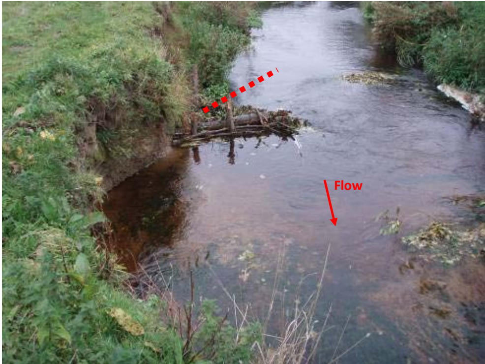
Photo 15 Repositioning this flow deflector to point more upstream will avoid the bank erosion currently occurring.
