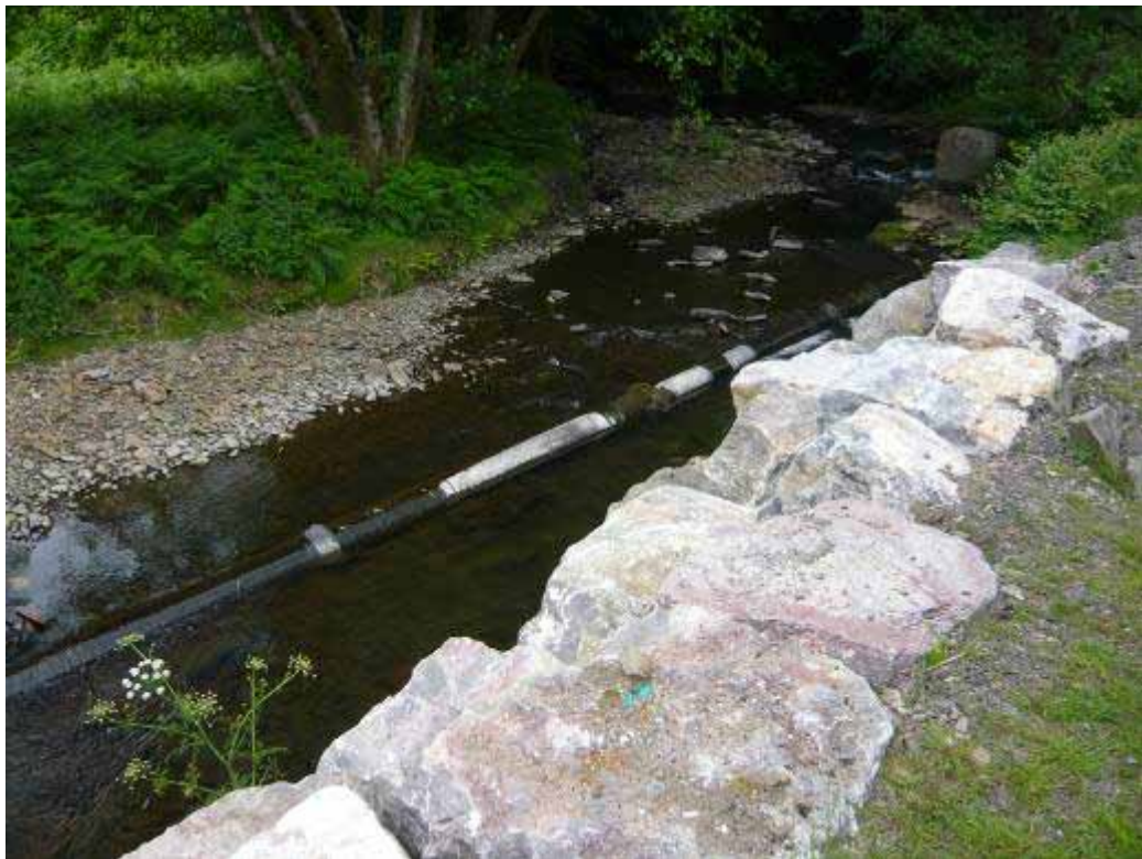
Exposed service pipe on the Ogwrfawr. Some sections of pipe were undercut and unsupported. A potential threat if the service is still in use?
