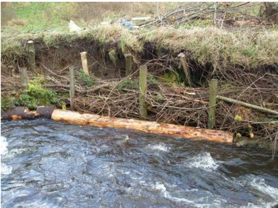
Work in progress. Tree trunk sections pinned to the toe of an eroded bank to be backfilled with wired down brush on the River Colne in Lancashire
