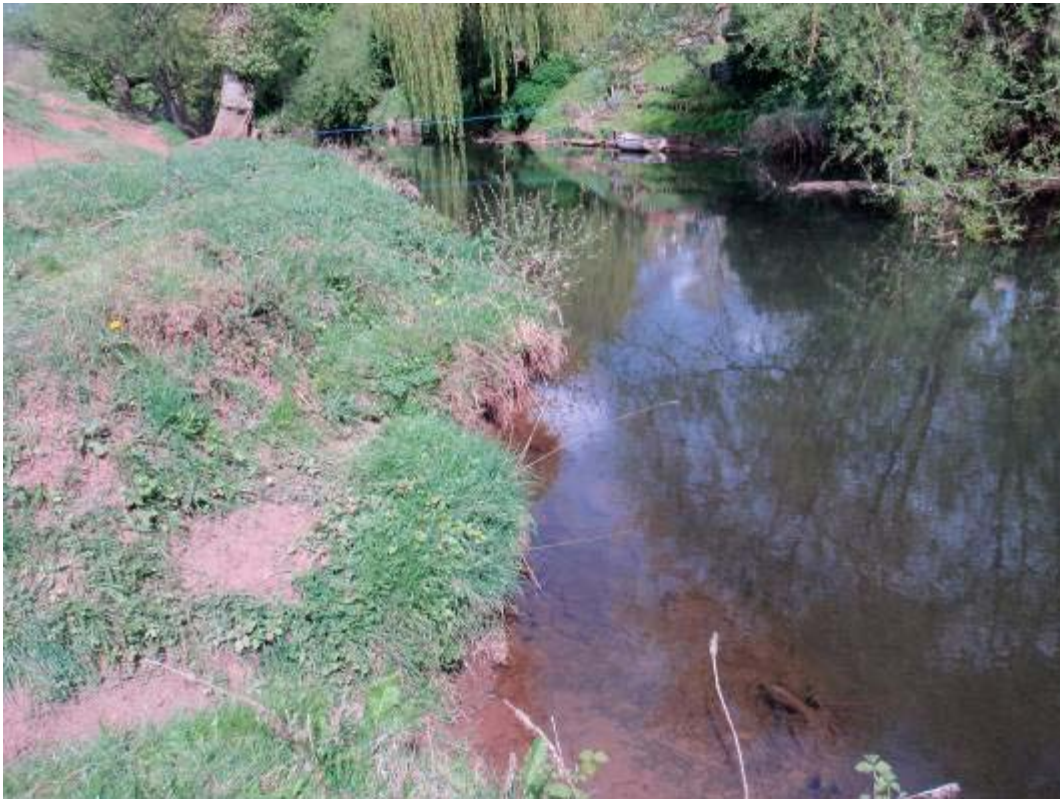
The toe of the bank is reasonably well vegetated and looks to be relatively stable
