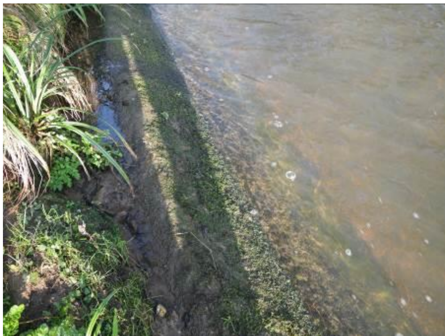
Photo 2. Battered concrete margin limiting the establishment of a natural river bank
