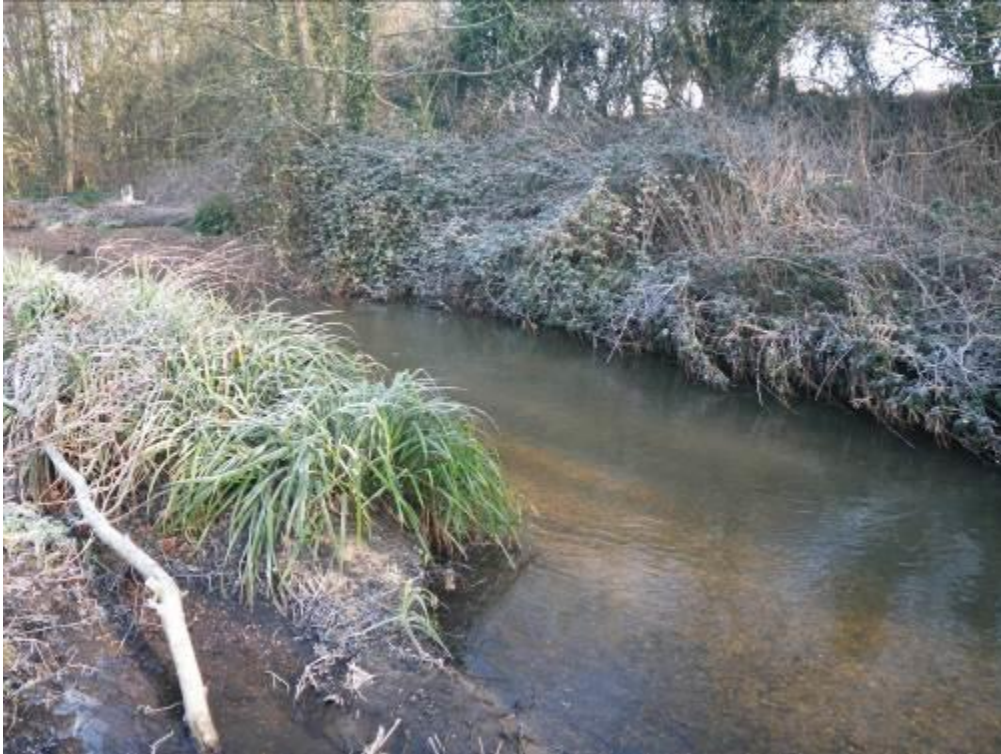
Photo 4. Bank sediments have been stabilized with the establishment of sedge beds. The overhanging bramble does provide a modicum of cover for fish seeking refuge during migration.
