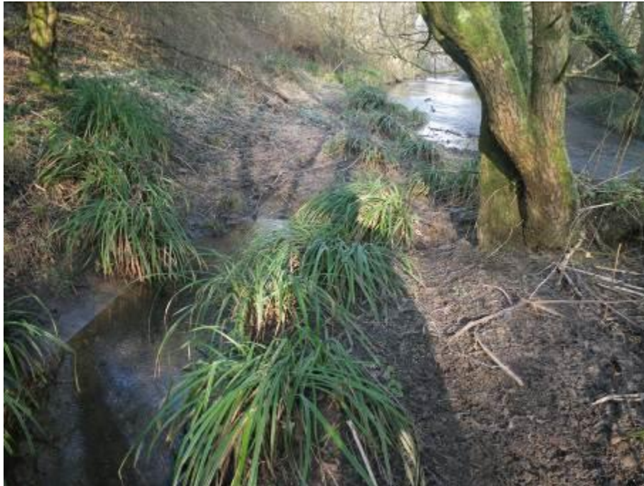
Photo 1. Sedge and even the odd shallow rooted tree have established on deposited river bed material. Note the exposed concrete bank on the left hand side of the photo.
