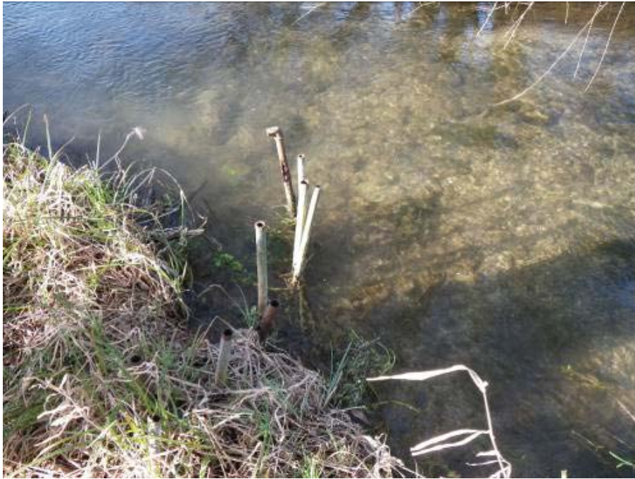
A line of old steel pipe that probably supported an old flow deflector which was commonly made from corrugated tin. A tree trunk pegged in at right angles to the flow and secured with a chestnut cleft would be an acceptable alternative.
