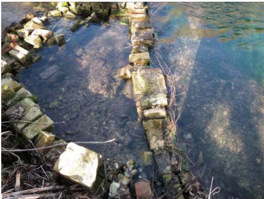
The remains of an old flow control structure. This section of bank should be repaired with a small notch to provide a very small sweetening flow to continue down the channel to the left.
