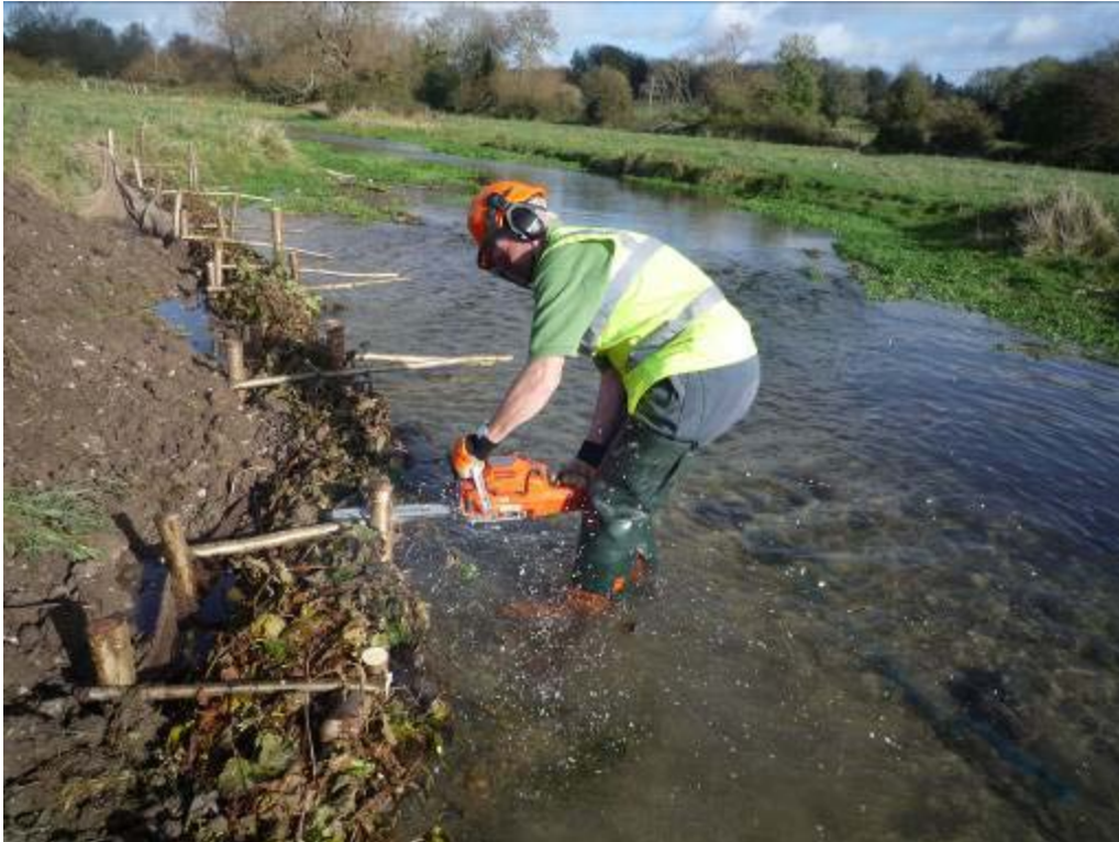
Installing a new faggot revetment on the Meon. The soil infill must be protected with a geotextile soilsaver to reduce the risks of the material getting washed out before planting becomes well established
