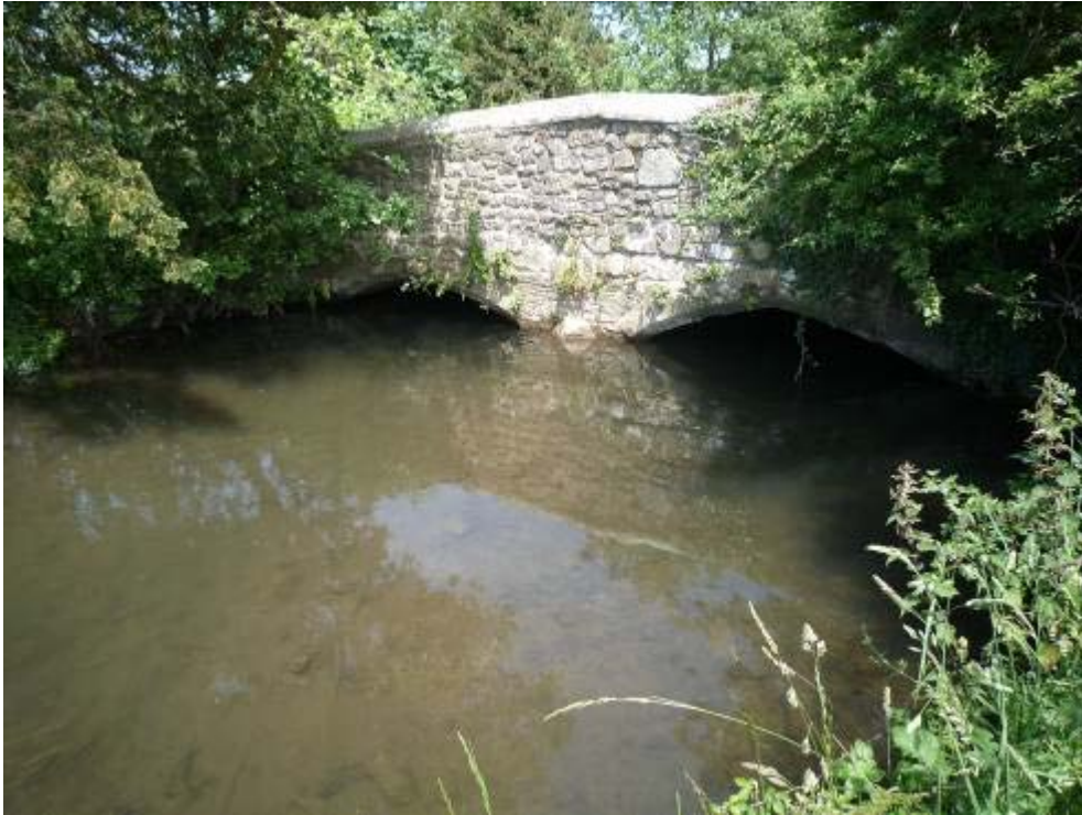
The small arches of the Anjou Bridge probably impound the river in the meadow above.
