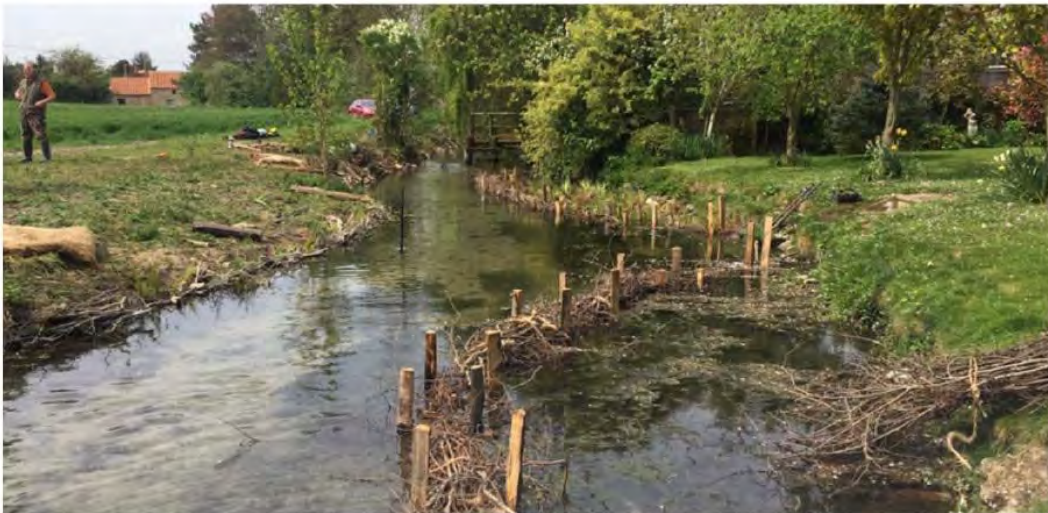
Photo 15 Installation of low level brushwood berms (before, above; after, below). Note the bank on the left of the picture, which has been re-profiled to a shallower angle to tie in with the new bank toe created by the brushwood bundles.
