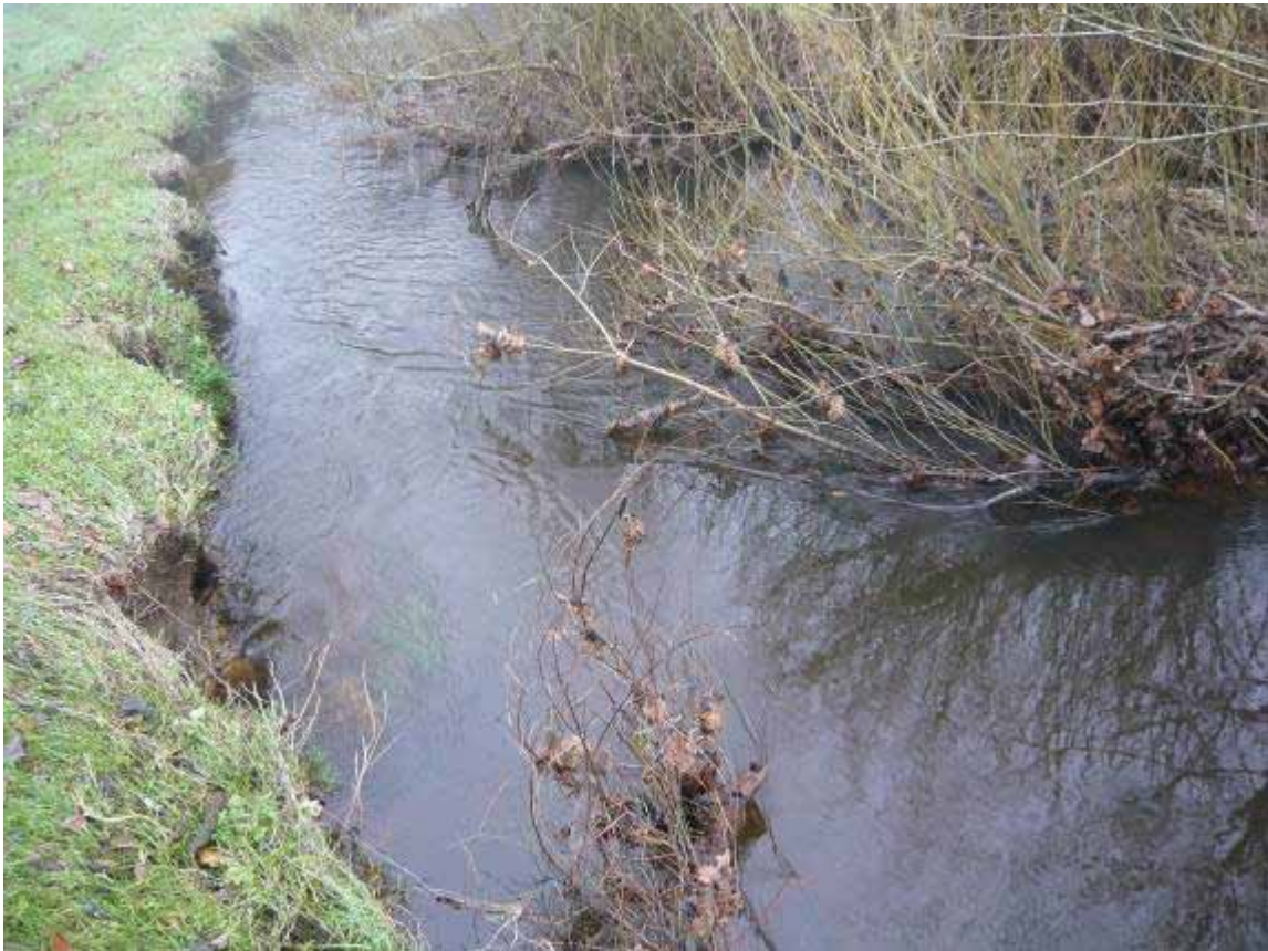
Light bankside erosion exacerbated by the encroachment of a line of willows
