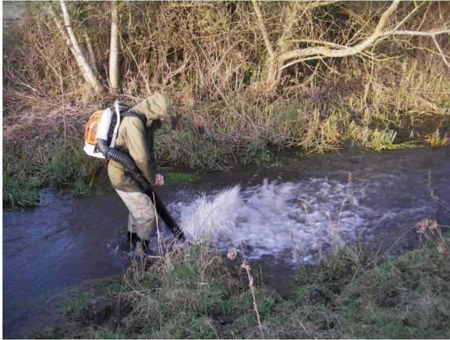
Gravel cleaning using a back pack leaf blower. Cleaning gravels on the very top section is recommended
