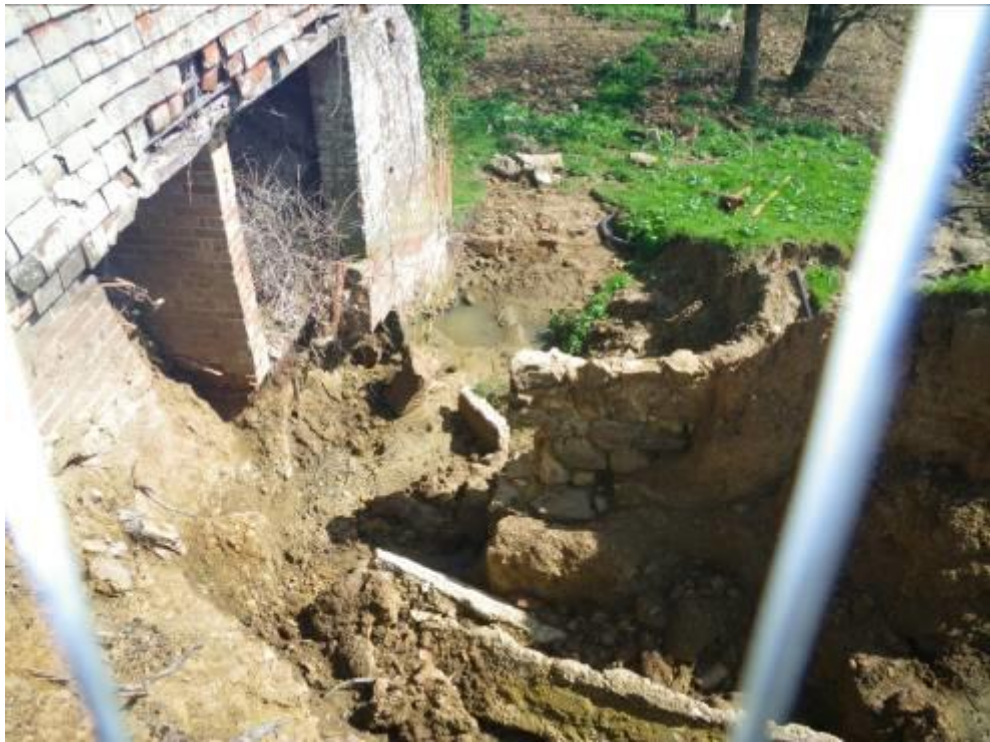
Photo 6. Damage to the downstream face of the dam.
