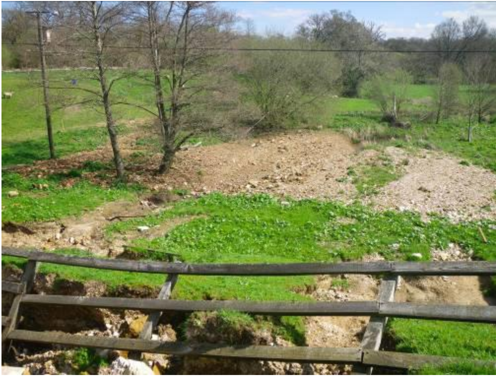
Photo 7. Spoil blown out from the dam structure.
