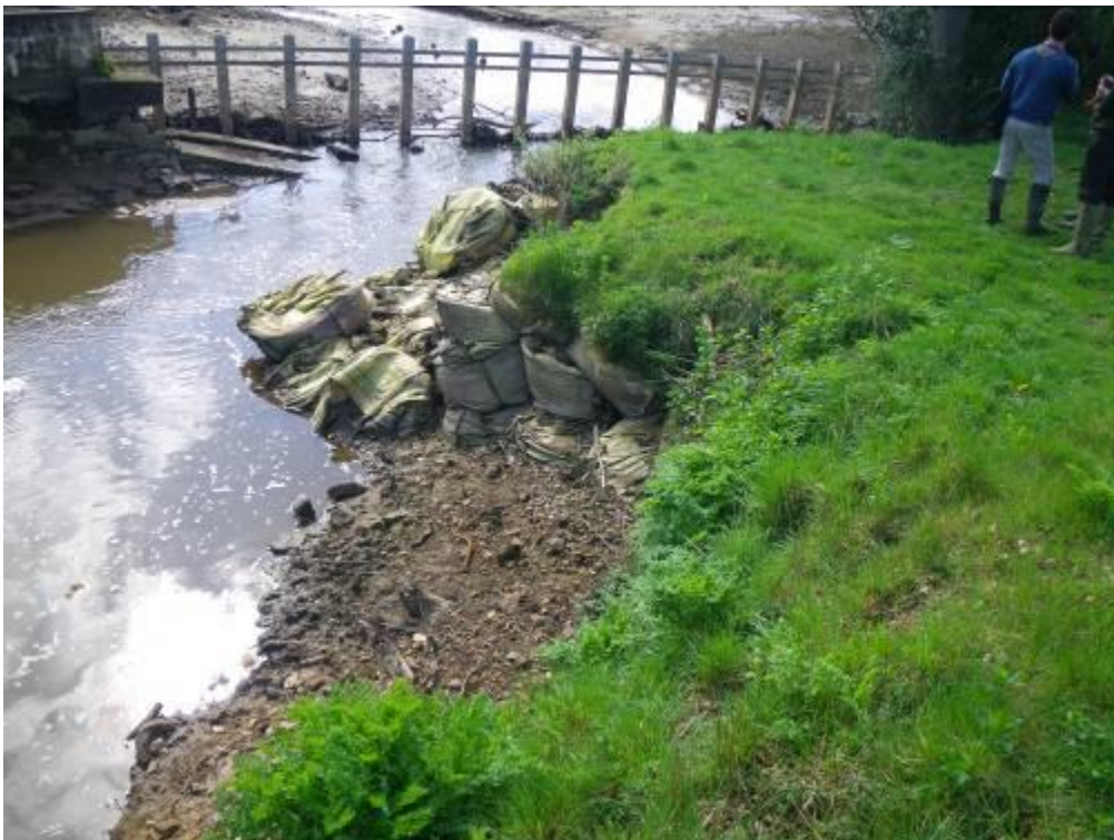
Photo 2. The trash screen/walkway should be removed, as should the temporary bank repairs. This area of bank will naturally recover.
