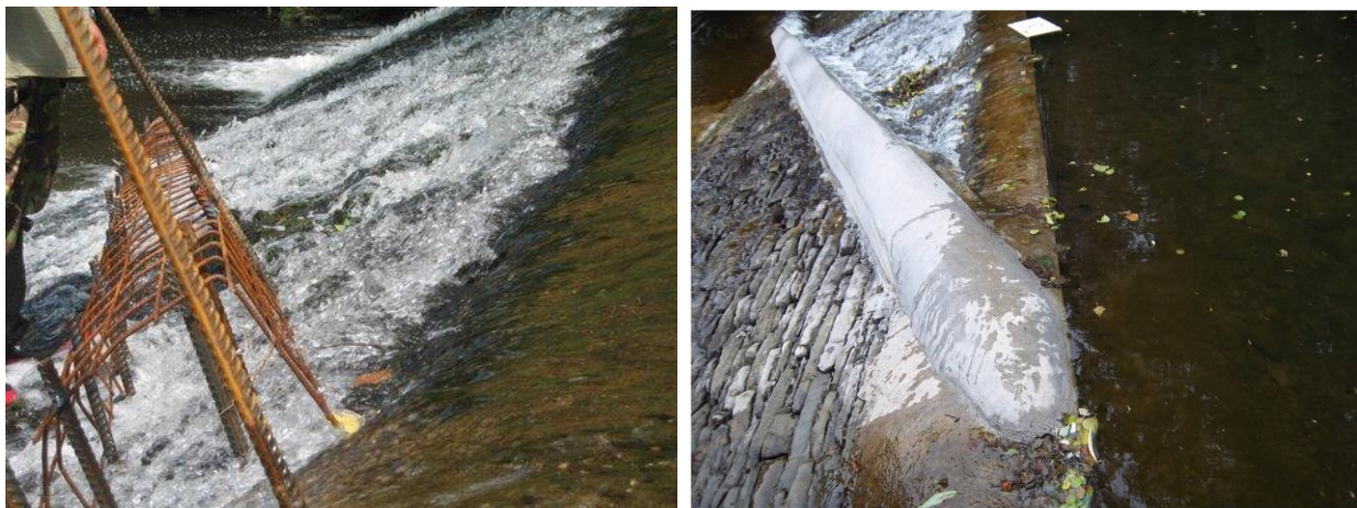
Figure 3: Concrete diagonal baulk (right) cast over rebar frame (left) courtesy of the Wye and Usk Foundation
