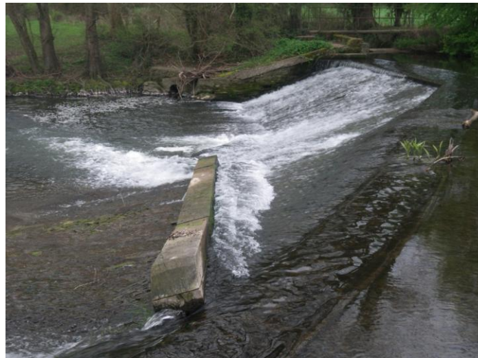
Figure 6: Wooden sleeper diagonal baulk easement – here the face of the weir is sufficiently uniform as to hold up a sufficient depth of water for fish to swim up without requiring additional sealant measures. Sleepers are attached by means of expansion bolts fitted into drilled recesses in the face of the stone-work. Courtesy of Wye and Usk Foundation.
