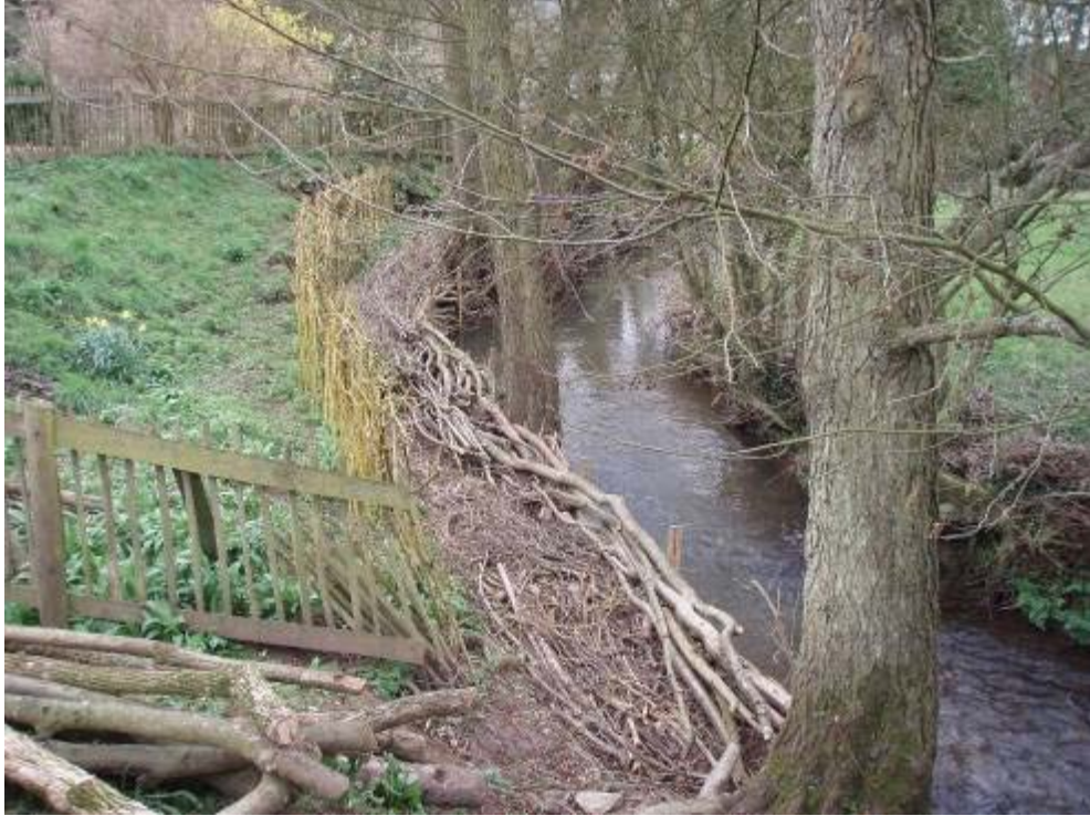
Photo 5 Bank revetment work using local brushwood – good erosion control and valuable habitat
