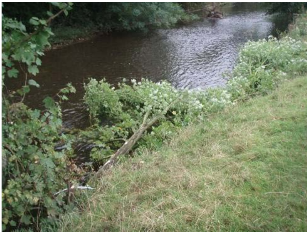
Photo 13 Whole tree anchored alongside the bank with steel cable to a standing tree (River Goyt, Cheshire)
