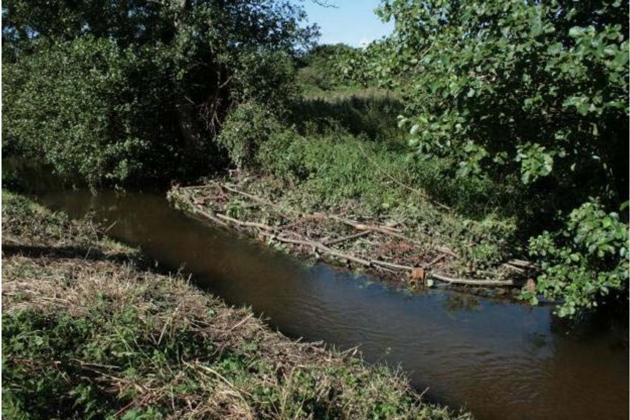
Photo 14 Brushwood mattress constructed to narrow the channel, provide juvenile fish cover and promote depth variation
