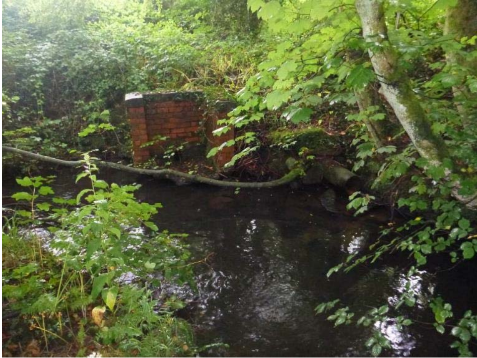
Photo 9 Headwall from a surface water drain. Clear demarcation of these at their source can assist in pollution prevention (for example by preventing spills being flushed down).
