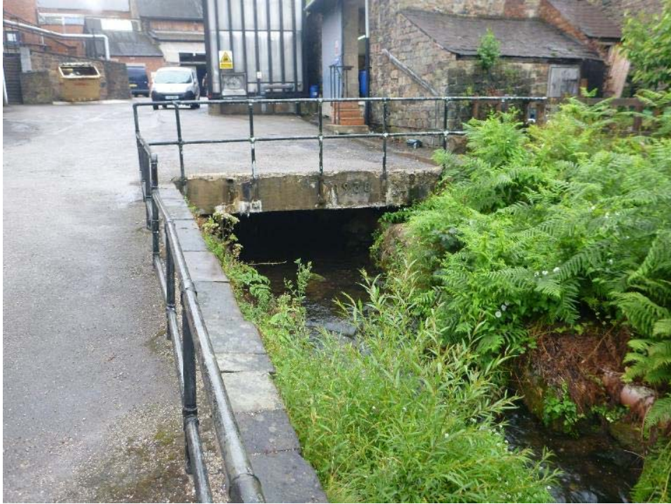
Photo 12 Downstream end of the factory culvert. The gradual transition from light to dark provided by the vegetation is better than an abrupt change in encouraging fish to pass into the culvert.
