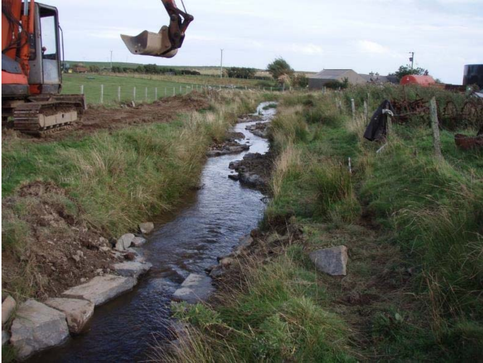
Photo 21 Stone structures built to improve depth variation without causing flow impoundment on a small burn on Orkney.
