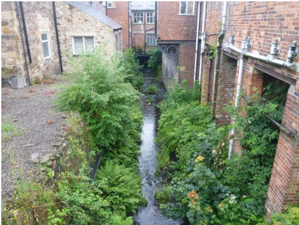
Photo 13 The upstream end of the factory culvert. The same comments as above apply. Also, the natural bed is far better than a smooth artificial surface (like concrete), assuming this extends the full length of the culvert.
