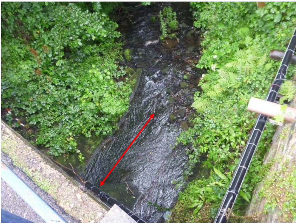
Photo 15 Upstream end of twin pipe culvert, showing extent of concrete base and shallow, fast water.
