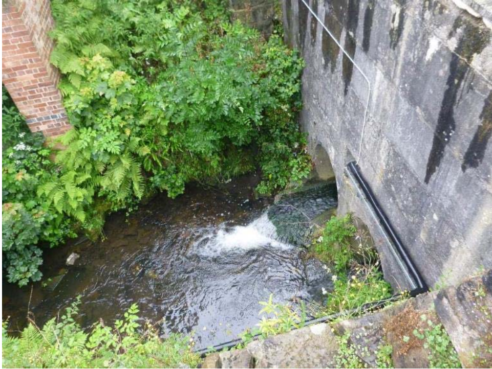
Photo 14 Above the main culvert under the factory, the brook is crossed by a bridge with a twin pipe culvert. The downstream end is perched above bed level. Along with the thin skim of water over the concrete bed of the pipe, this creates an obstacle to fish passage.
