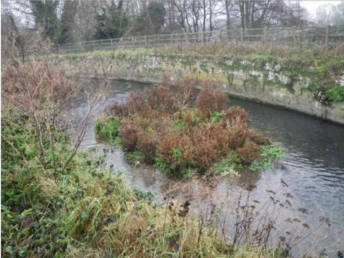
The old cutting where tree cover has been removed, presumably to protect the integrity of the wall
