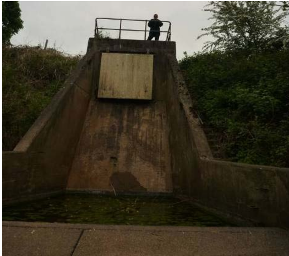
Figure 5: Large Combined Sewer Outfall (CSO) at NGR: SD 76551 04705
