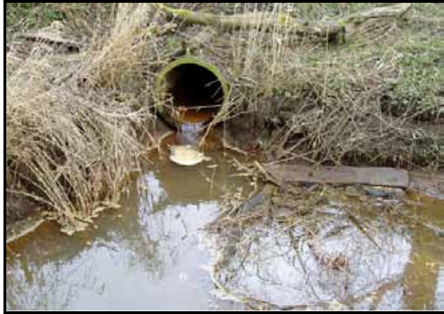
Plate XV: Seepage pipe from covered landfill site
