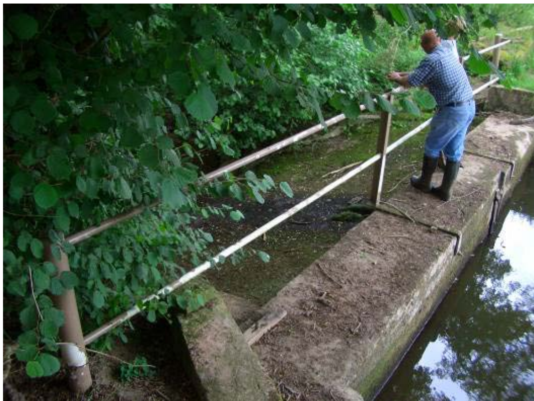
A massive concrete weir fragmenting populations and habitat on the How Capel Brook
