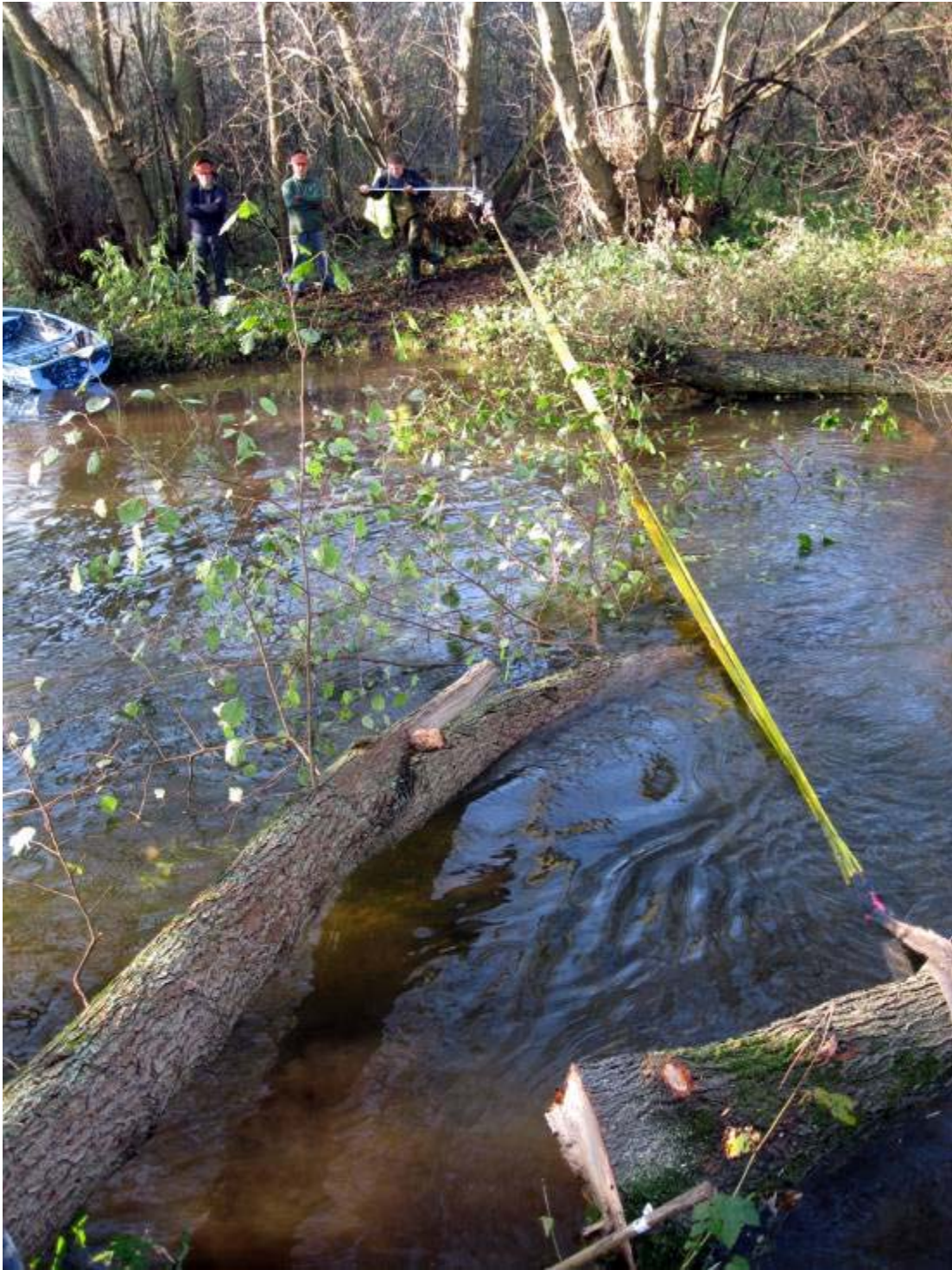
Photo 23 Work in progress installing large woody debris on the River Bure, Norfolk.
