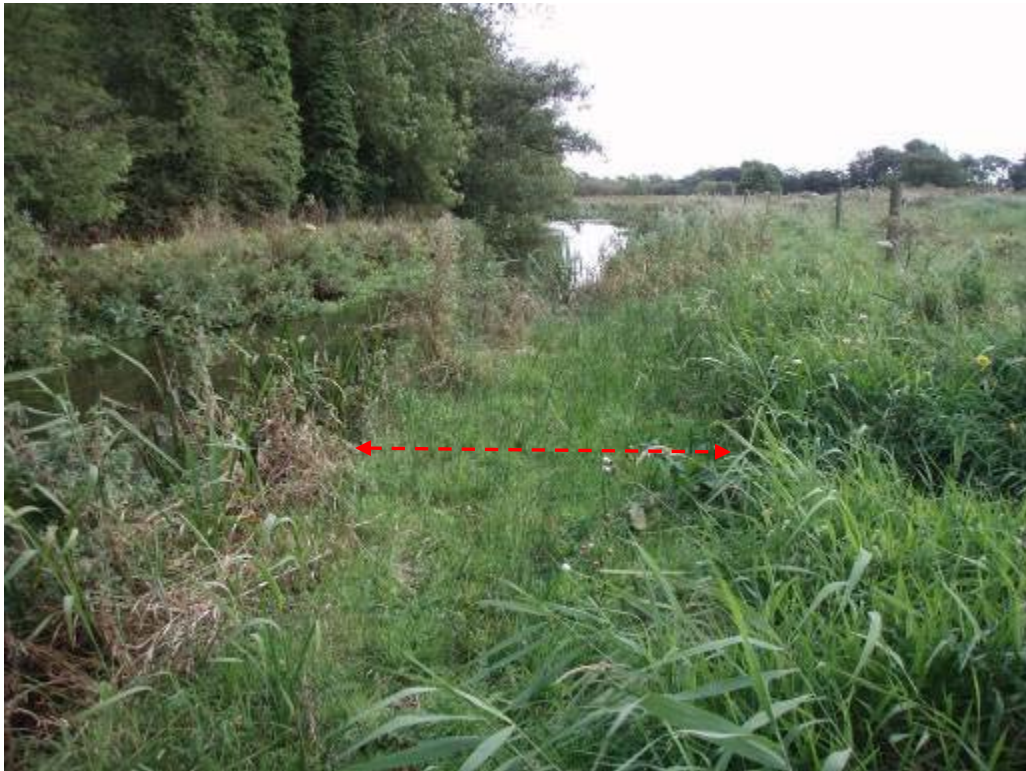
Photo 20 Low berm created to narrow the channel, using brushwood bundles and backfill.
