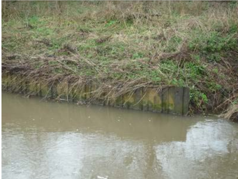
Hard revetment and no cover – a hostile environment for trout
