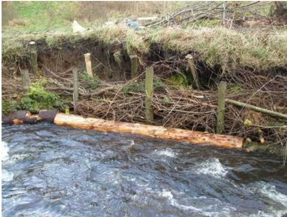
A brushwood mattress installed adjacent to an eroding bank on a spate river. A variation of this technique could be used on the Fynn.
