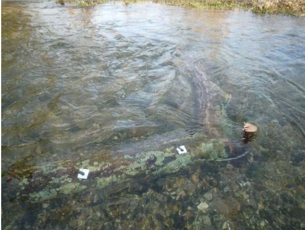
A small upstream "V" deflector pegged onto a shallow chalkstream glide and designed to promote movement of bed material.
