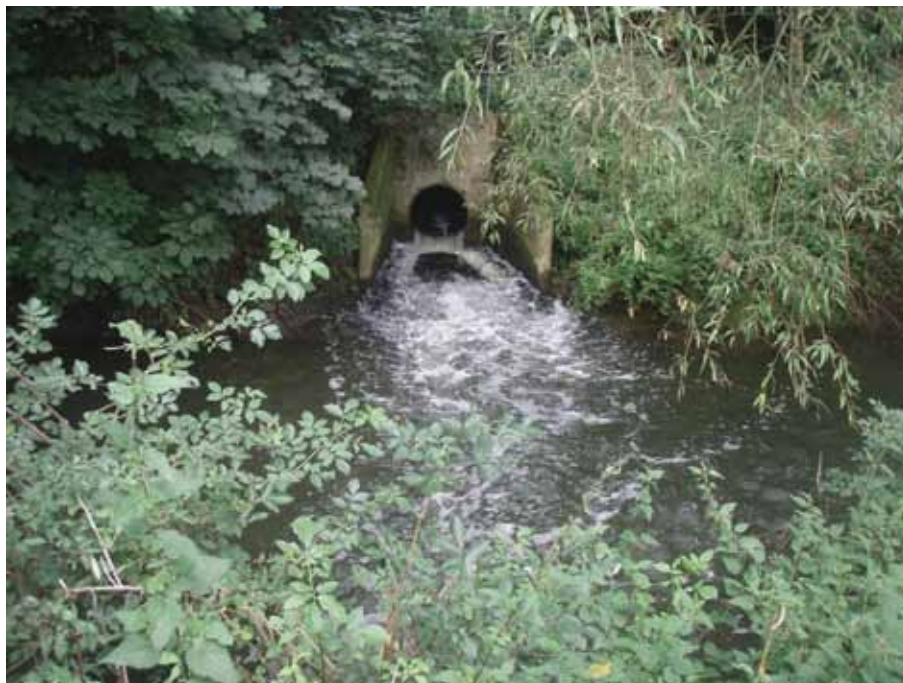
Photo 9 Hallam Fields STW outfall
