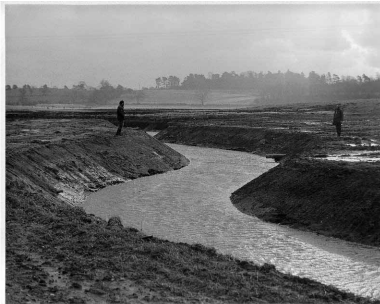
Photo 11 An example of 1970s river engineering works creating an incised channel with a trapezoidal cross-section and the loss of pool and riffle habitat structure (River Sow, Staffordshire).
