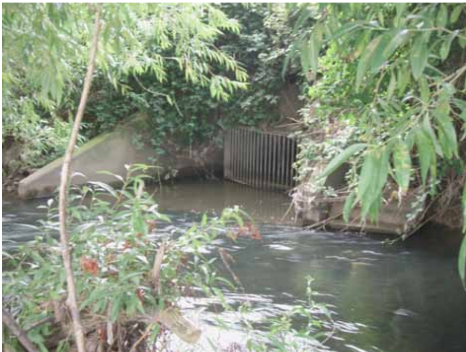
Photo 2 Combined Sewer Overflow (CSO) discharge point on the River Erewash
