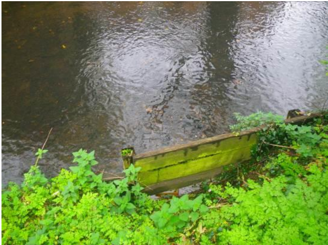
Photo 4. Toe-board failure adjacent to the LB was evident in several locations.
