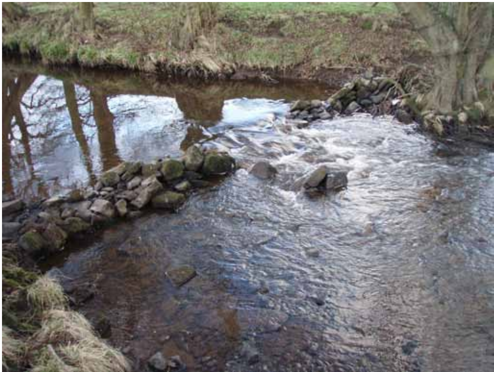
Photo 14 Weir constructed by UDFP to retain water levels and depth for adult trout (the centre has collapsed). A design to promote downstream scour, rather than retain upstream depths, would be better.
