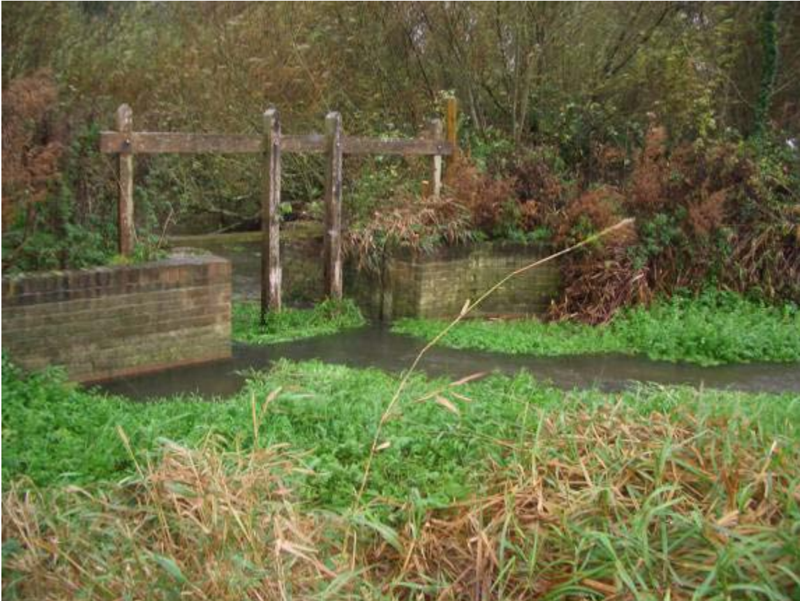
Structure responsible for impounding the reach that runs in front of the main farmhouse
