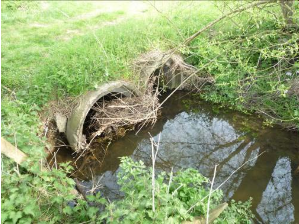
Blockage on the upstream end of the stream culvert. An open channel and clear span bridge may encourage fish to run the stream.
