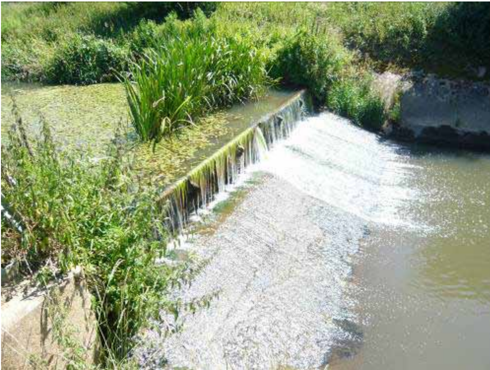
Environment Agency weir near the bottom boundary of the fishery. A barrier to fish migration during low flows
