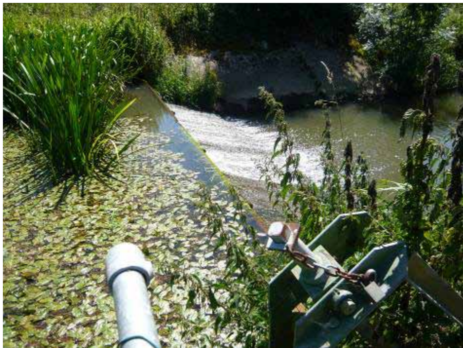
This old structure holds the key to improving fish migration and habitat quality
