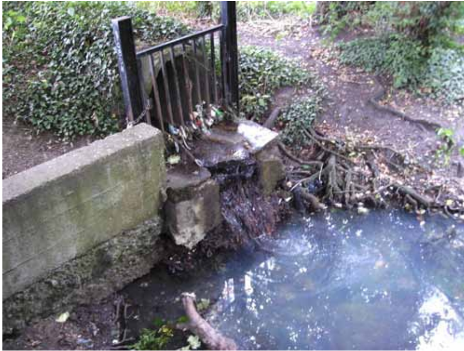
Photo 7: Last remaining problem effluent discharge on the Cray.
