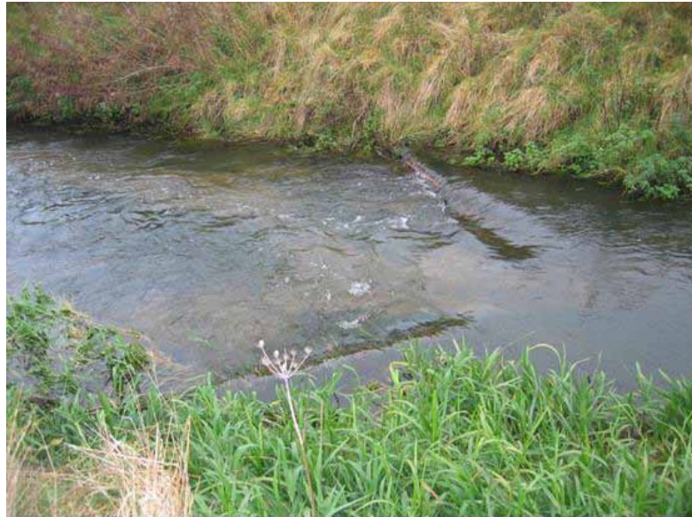
Figure 2: Paired upstream facing flow deflectors generating mid channel scour
