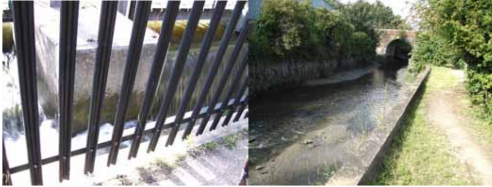
Photo 18: Vitbe sluice (left) and the tidal reaches of the Cray below (right)
