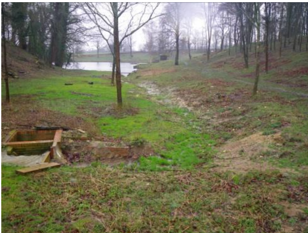
Figure 2. Inlet channel lost in a culvert.
